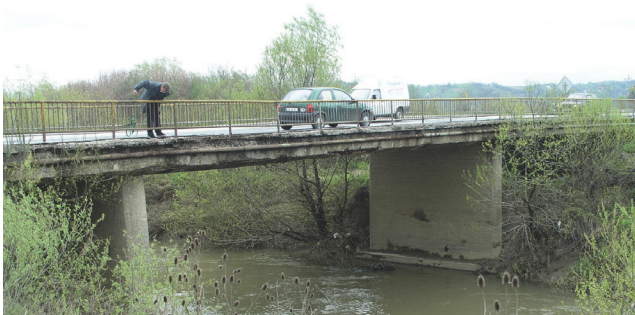
Figure 1. Bridge managed by Hrvatske ceste prior to repair in 2012 – typical damage to cornice and superstructure
