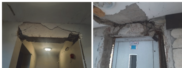
Figure 23. Examples of short-beam cracks connected to elevator shear walls
