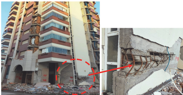
Figure 19. Plastic deformation and out-of-plane bending damage in Iskenderun–Hatay shear wall
