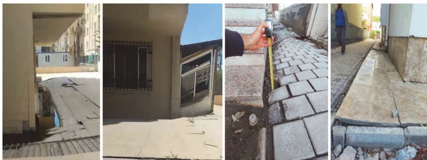
Figure 11. Approximately 60 cm subsidence and some settlements detected in Iskenderun after the earthquake
