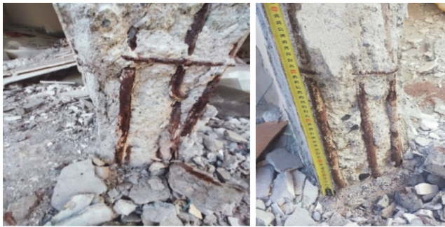
Figure 18. Loss of concrete reinforcement adherence and thinning of reinforcement diameter (cross-sectional loss)
