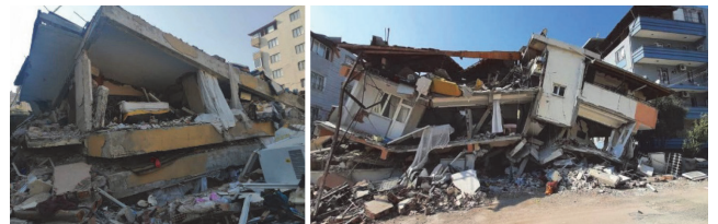
Figure 21. Strong beam-weak column behaviour in Antakya and Iskenderun
