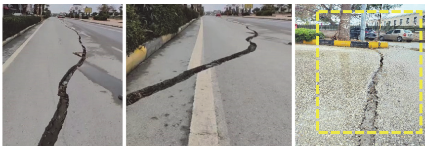
Figure 10. Settlement damage detected along the Hatay coastline
