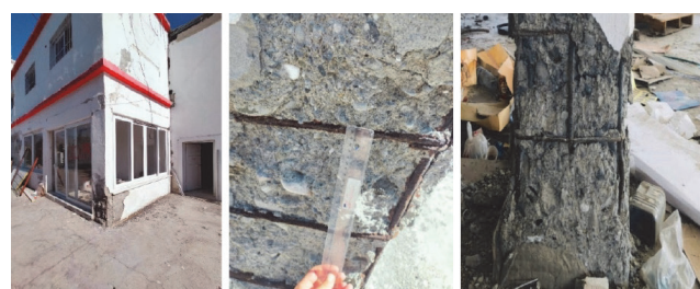
Figure 17. Structural defects in a damaged multi-story building in Hatay after an earthquake
