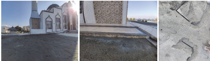
Figure 9. Highway cracking in Hatay
