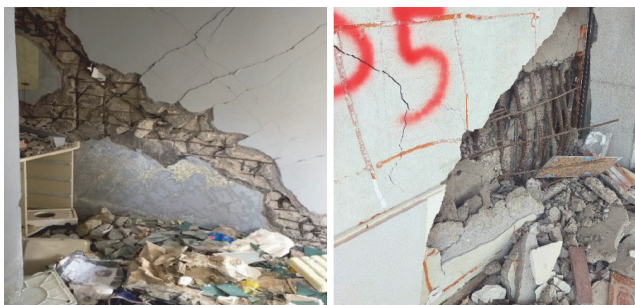
Figure 20. Diagonal cracks and loss of sections in structural walls
