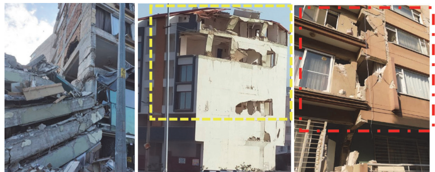
Figure 13. Buildings whose structural elements were damaged by adjacent constructions
