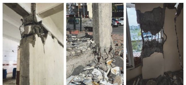
Figure 22. Inadequate transverse reinforcement
