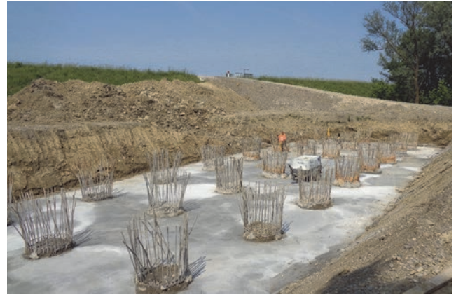
Figure 5. Pile heads and blinding concrete for pile cap at pier position S6, B&H side
