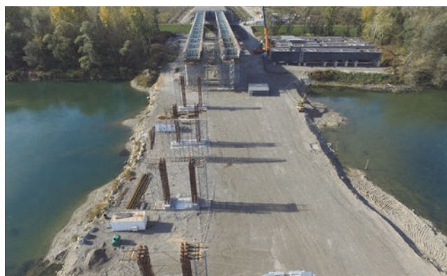
Figure 8. Completed steel structure up to pier S5, platform with macro-elements and temporary supports between piers S5 and S4, Bosnia and Herzegovina side
