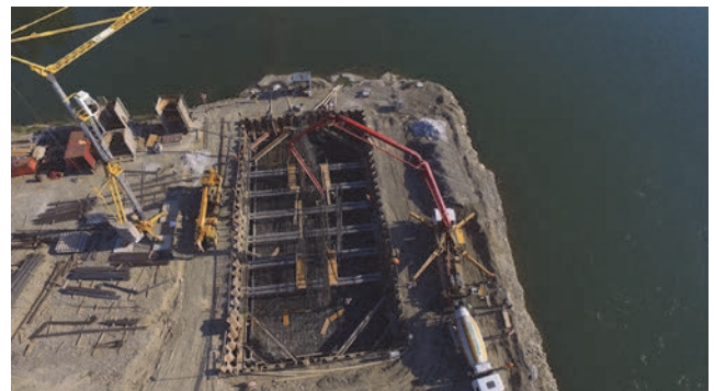
Figure 6. Foundation pits at pier position S3, Croatian side, with pile cap reinforcement already in place
